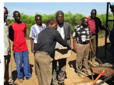
Laying of the church cornerstone by Rev. Lazarus Mbewe and Robert Nkunika, Clerk of Session, while left background shows two building contractors and three members of the church vestry in dress shirts L-R; Frank Muwowo, Julius Chihana and Peter Banda (85-yrs of age)
